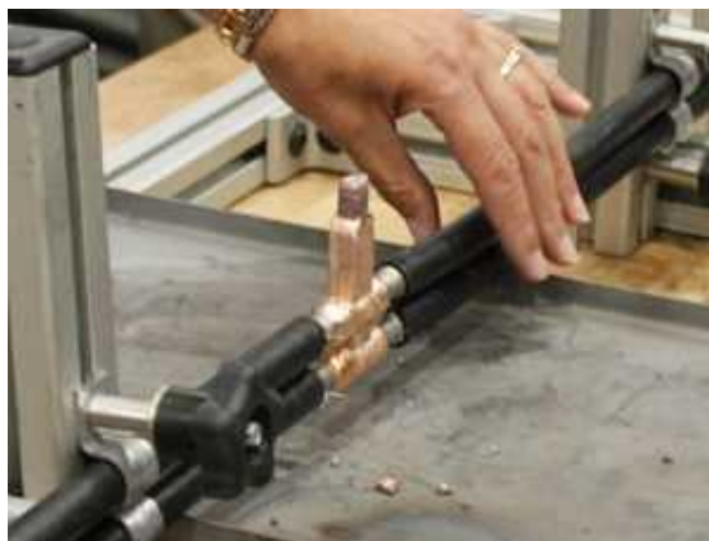
An exothermic welding process has been validated for use on CVN 78. NMC photo
