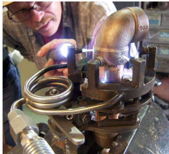
Shipbuilding costs are being reduced by brazing pipe joints with a small, lightweight heating system as opposed to using a hand-held torch. This NNS photo shows the first CVN 78 production pipe being brazed using the new technology.
